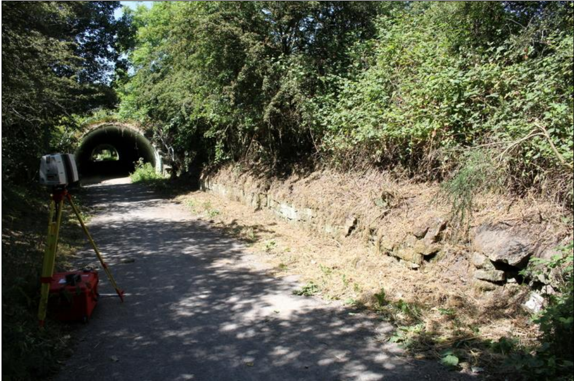
Plate 5: General view of the cleared element of the northern retaining wall, looking north-west
